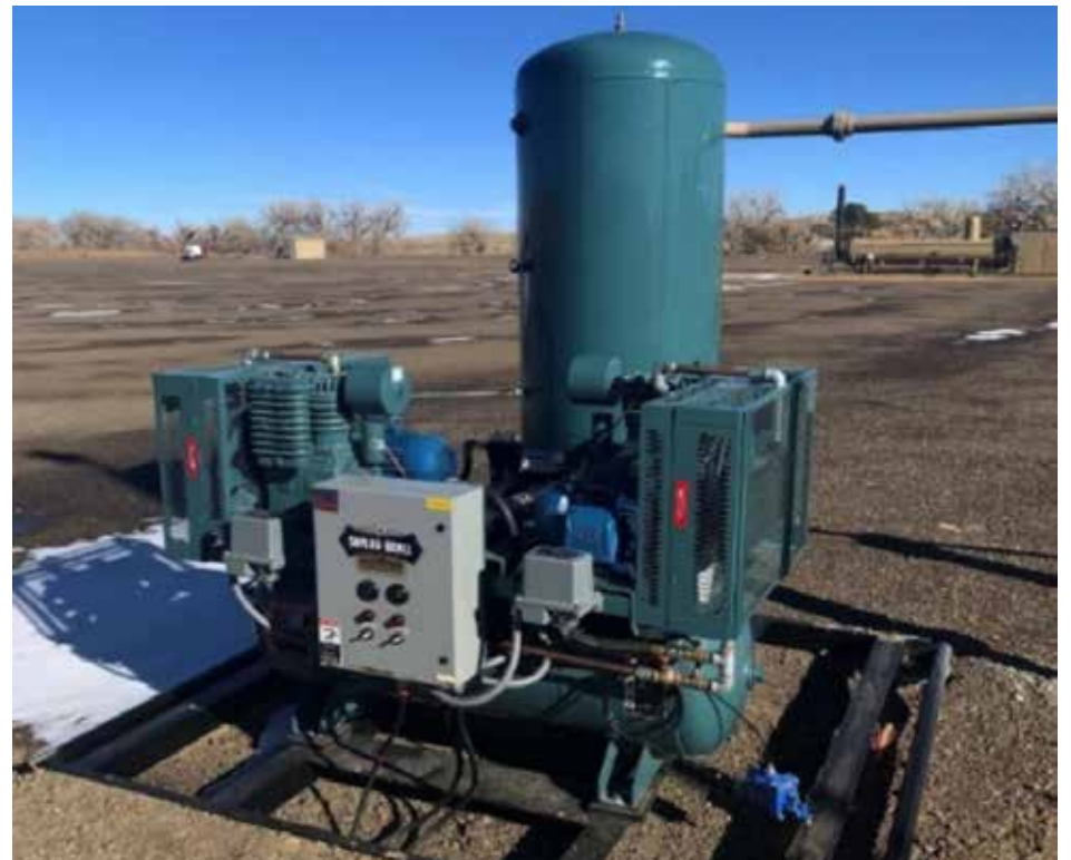
Figure 1: Skid mounted packaged compressor. Photo courtesy of VanZandt Controls.
